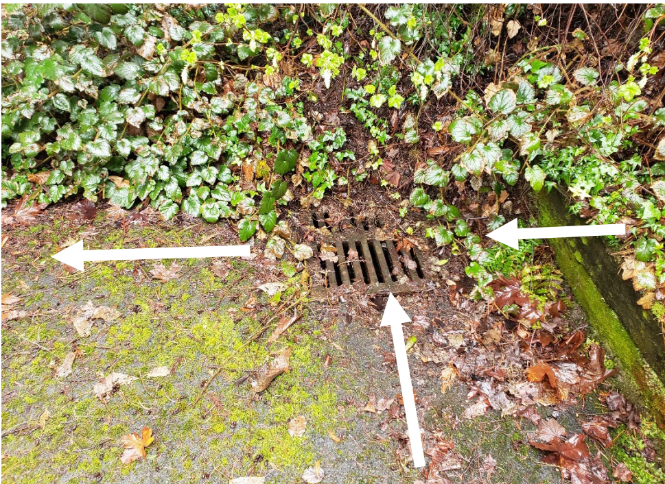
Photo 6. Stormwater catch basin 29-124 with flows toward conveyance channel to the north (arrows for direction of flow).
