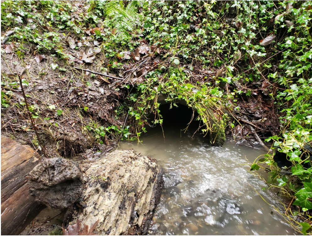
Photo 9. Stream A flows into 24-inch concrete culvert, a segment of piped stream flowing northwest toward Lake Washington.
